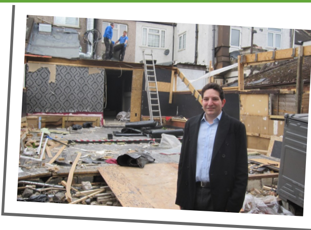
Cllr Stephen Greek inspecting a potential site contravening planning regulations.
